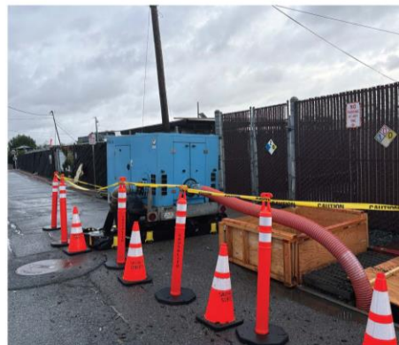
City's temporary pump installation on Gate 5 Road
