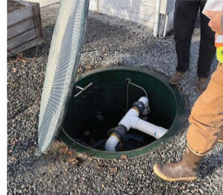
Private property sump pump system
